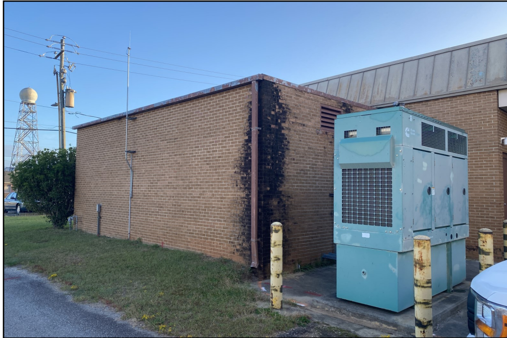
Figure 1: Southwest view of Airfield Lighting Vault generator
