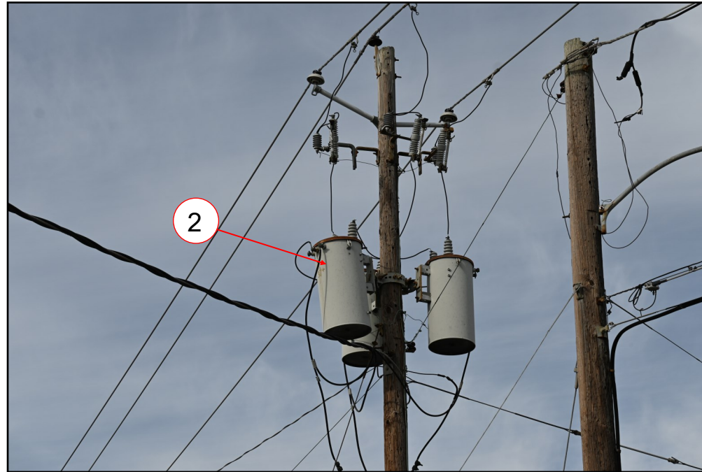
Figure 2: Local Utility transformers with 208/120 secondary furnishing existing FBO Terminal Building
