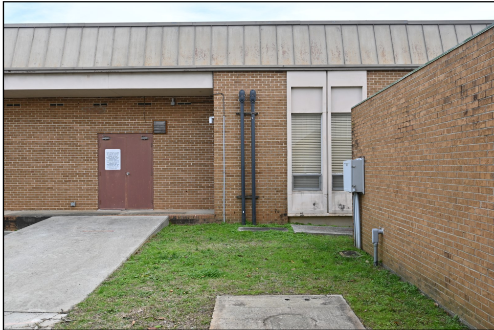
Figure 1: Twin 2" PVC conduits mounted on west wall of FAA Avionics Building
