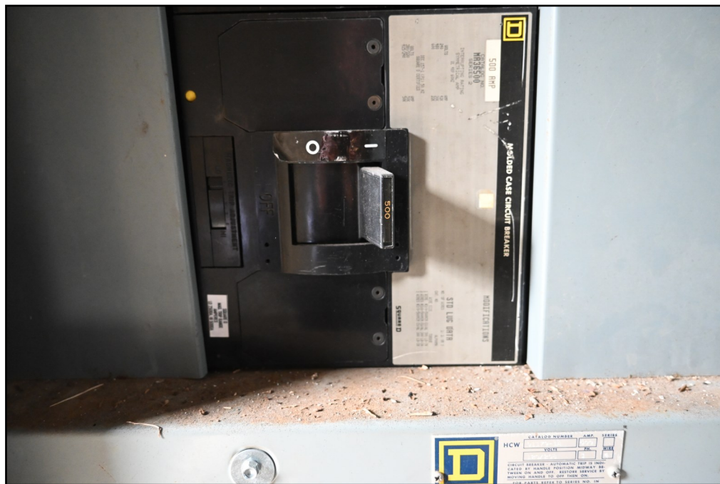
Figure 3: 500 Amp main circuit breaker in 208/120 Volt 3-phase switchboard
