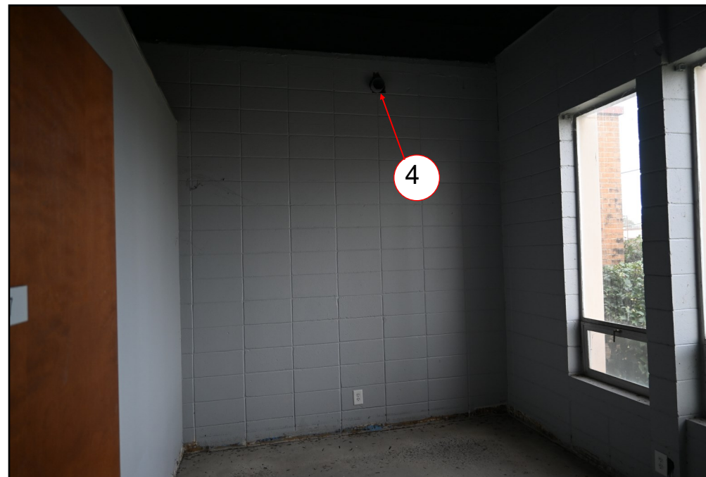
Figure 4: Termination of 4" PVC conduit (abandoned) in FAA Avionics Building from Airfield Lighting Vault
