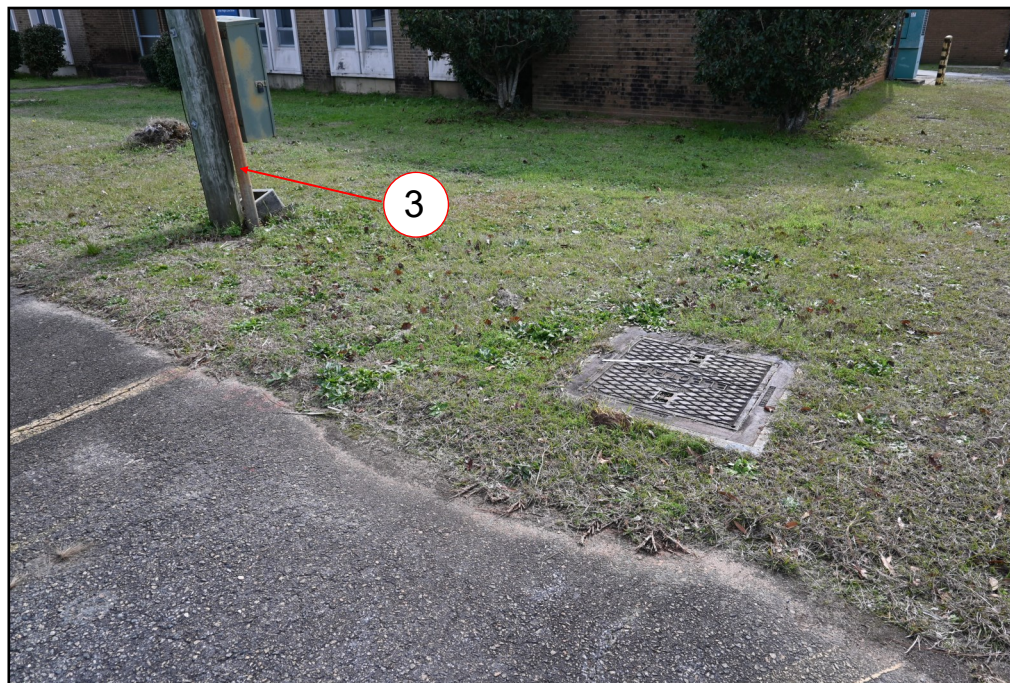
Figure 3: 2" Rigid conduit with 2400 Volt conductors to Airfield Lighting Vault
