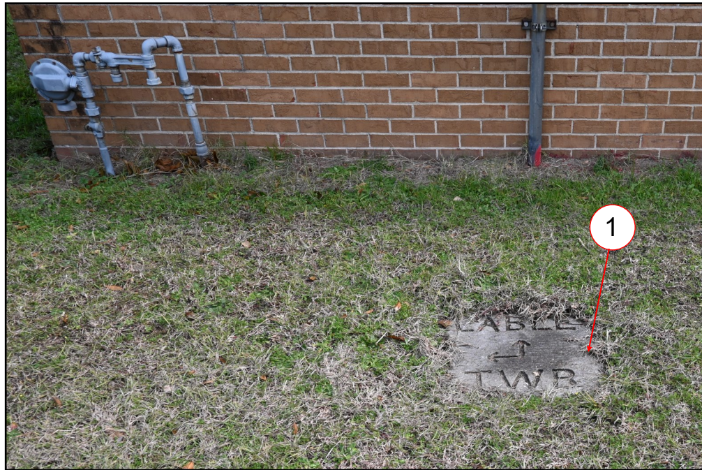
Figure 1: Airfield lighting cable marker adjacent to Airfield Lighting Vault
