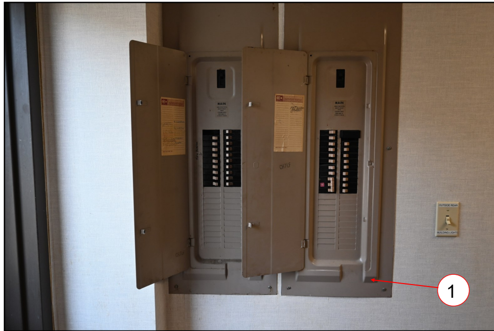
Figure 1: Twin 208/120 Volt, 200 Amp panel boards in existing FBO Terminal Building
