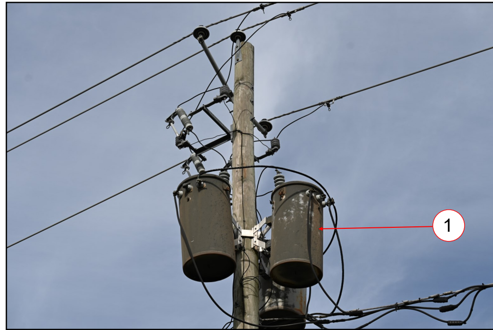
Figure 2: Local Utility transformers furnishing FAA Avionics Building
