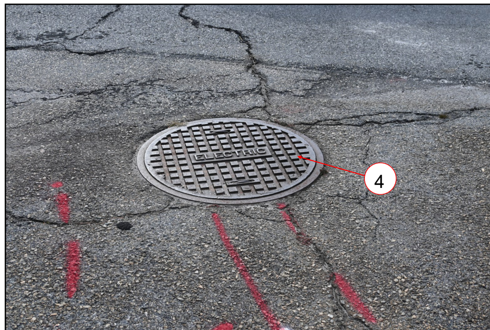
Figure 4: Airfield Lighting Ductbank junction structure at apron on south side of FAA Avionics Building
