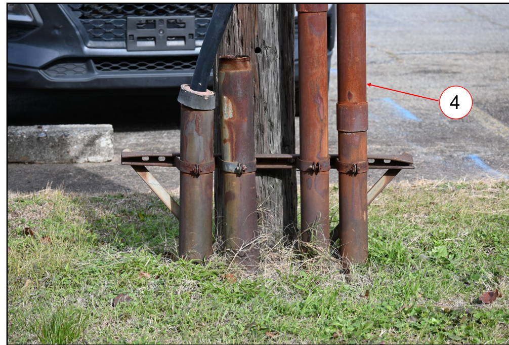
Figure 4: Utility transformer secondary feeders to main switchboard in FAA Avionics Building
