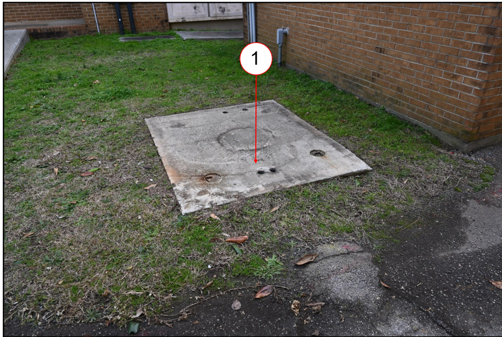
Figure 1: Abandoned electrical equipment pad
