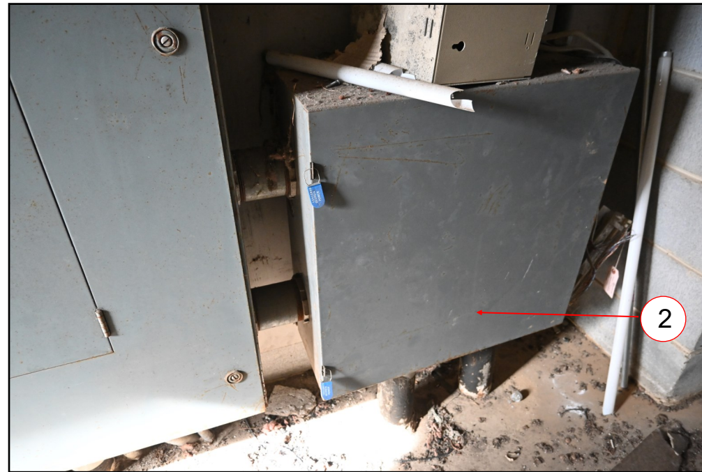
Figure 2: Pullbox, with Georgia Power lockouts, between incoming floor conduits and main switchboard
