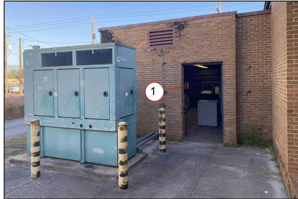
Figure 2: Southeast view of Airfield Lighting Vault generator
