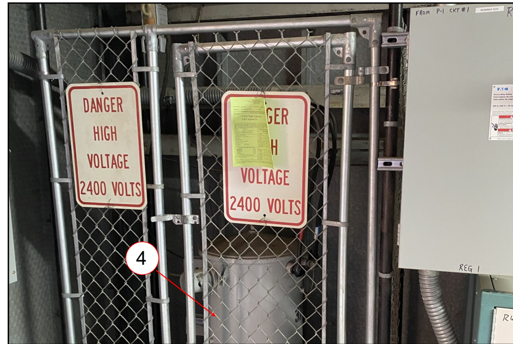
Figure 4: Airfield Lighting Vault incoming power transformer 2 of 2 (2400 Volt primary, 240 Volt secondary)
