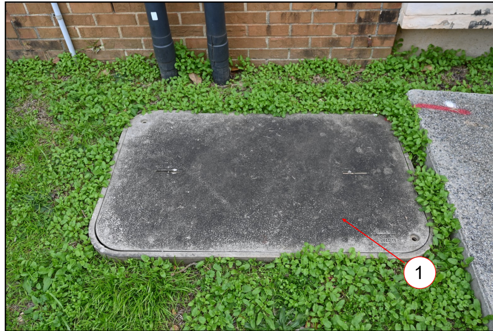
Figure 2: Polymer Concrete junction structure adjacent to conduits mounted on exterior wall of FAA Avionics Building
