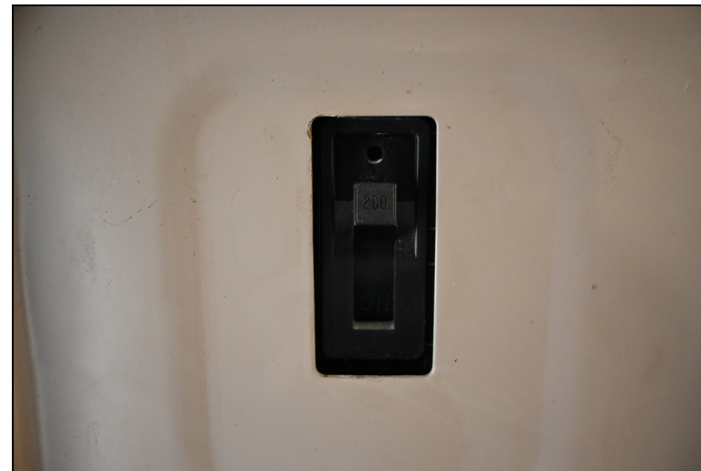
Figure 2: 200 Amp, 3 pole main circuit breaker for panel board 1 of 2 in existing FBO terminal Building
